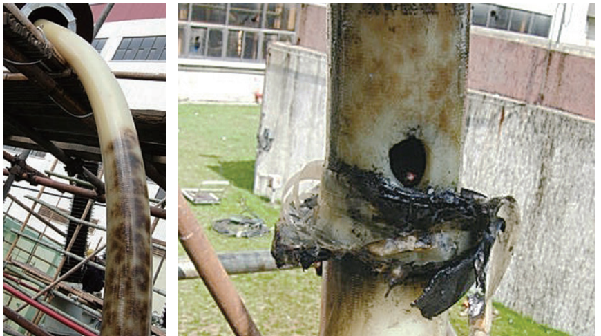
Figure 2. Left: Water tree caused by the interaction between the electric field and moisture. Right: Close-up of the mechanical damage to the insulation layer.
