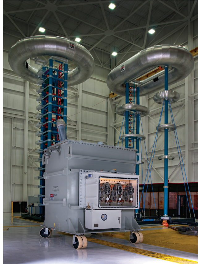
Vacuum Reactance Load Tap Changer at ABB's Alamo, Tennessee Facility.
