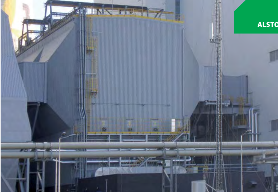
Figure 1. A recently commissioned Alstom electrostatic precipitator placed after an 850 MW lignite-fired boiler in Poland.
